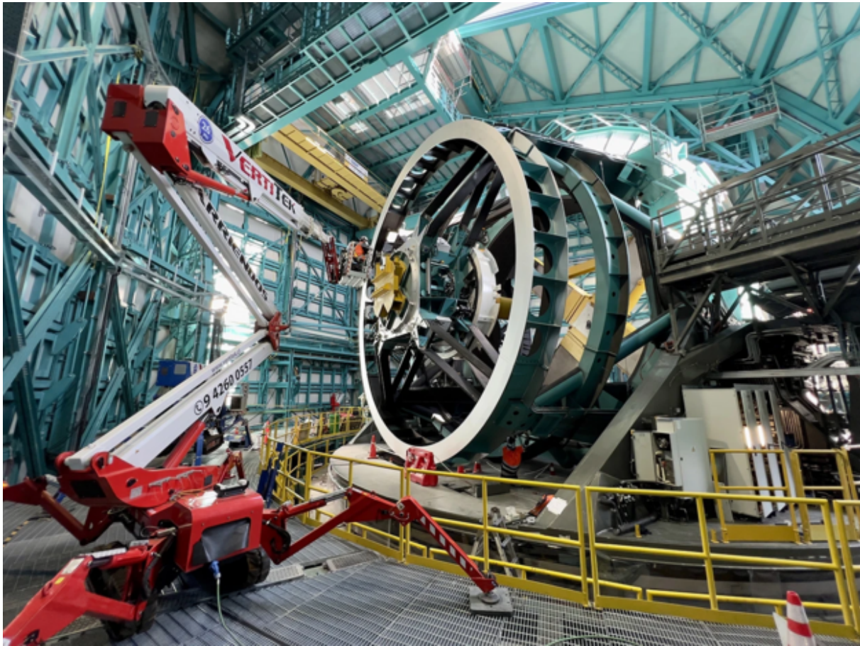
A technician installs fibre-optic cables at the Vera C. Rubin Observatory, which is due to take its first images in 2023. Credit: H Stockebrand/Rubin Obs/NSF/AURA. Preuzeto iz M. Naddaf, Nature 613 , 11–12 (2023).
